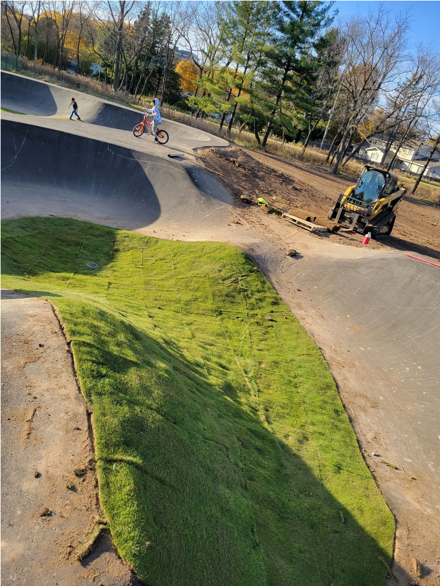
Infield SOD Photo 2
