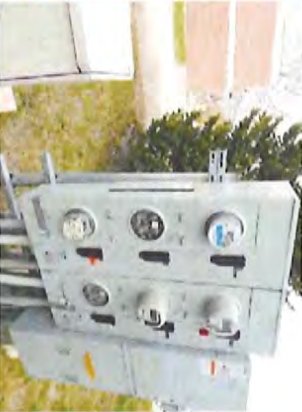
EXISTING METER BANK SCALE: NTS ⑦
