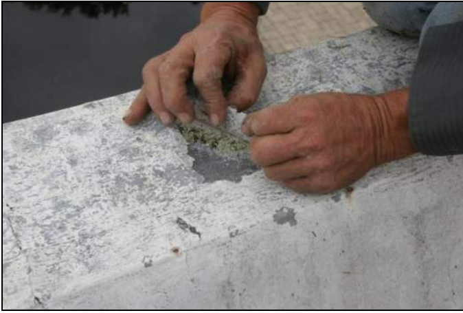
Fig. 5 – deteriorated lead flashing – loose pieces peeling exposing bare wood below
