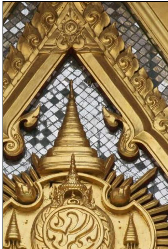
Fig. 8 – missing silver mirror squares (black squares). South-facing gable end of sala
