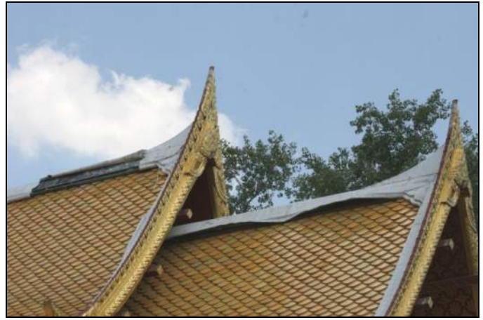
Fig. 2 – ridge roof flashing pulling away from tiles
