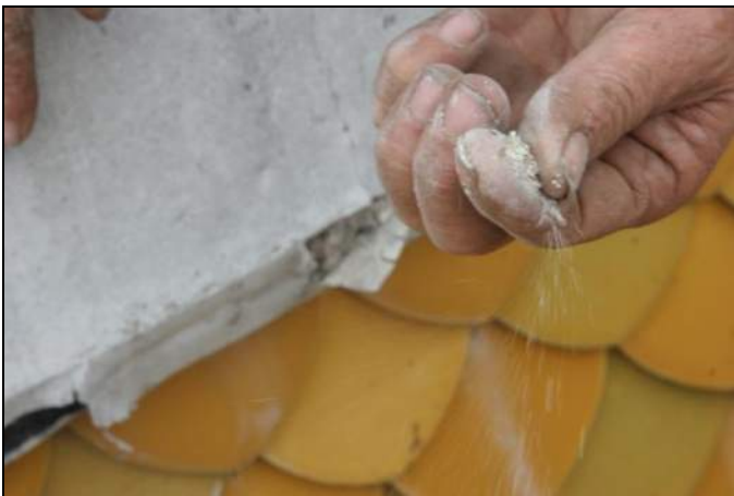
Fig. 7 – deteriorated lead flashing and paint
