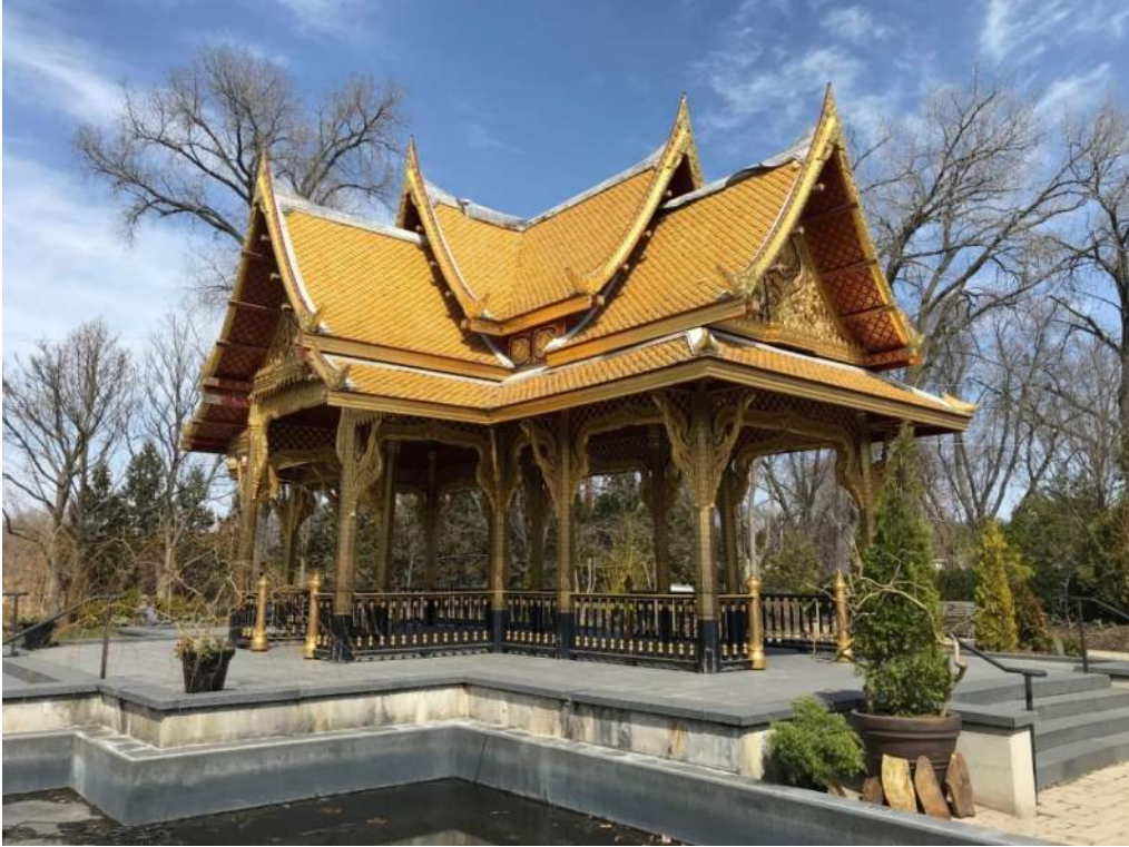
Condition of Thai Pavilion spring 2021.
