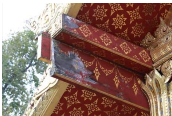
Fig. 20 – peeling paint – east side of sala
