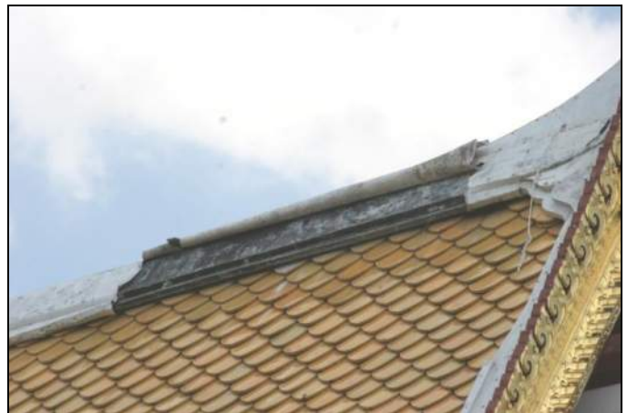
Fig. 3 – flashing curled and wood exposed allowing water to penetrate the attic and ceiling
