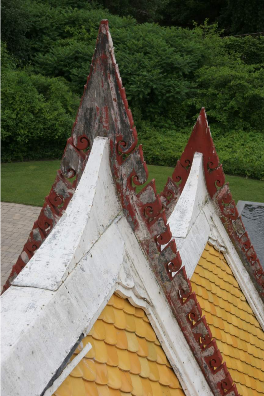
Thai Pavilion roof detail condition.
