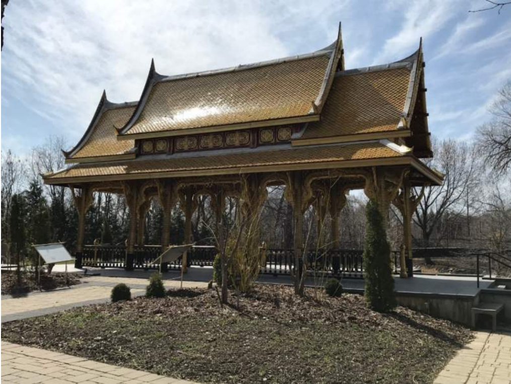
Condition of Thai Pavilion spring 2021.
