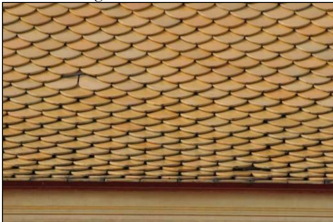
Fig. 1 – missing roof tiles need to be replaced
