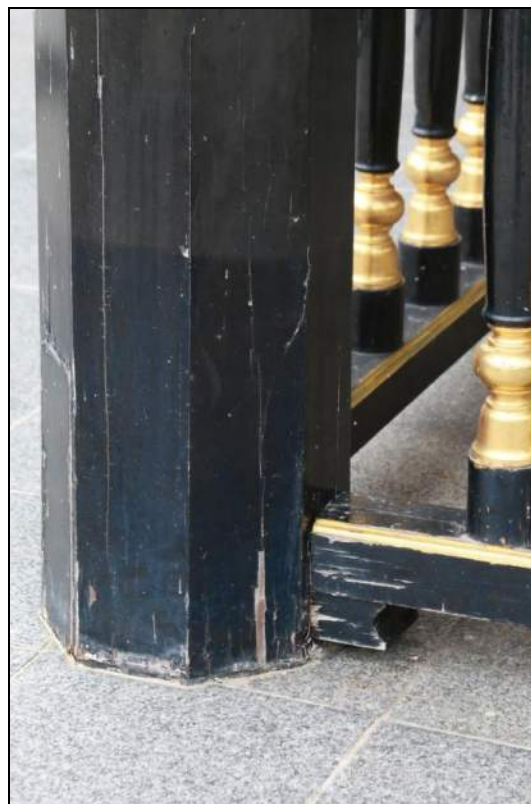
Fig. 12 – Column base – wood checking
