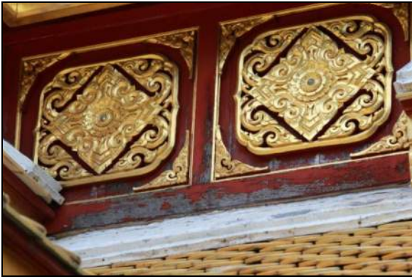
Fig. 23 – peeling paint on east side of sala
