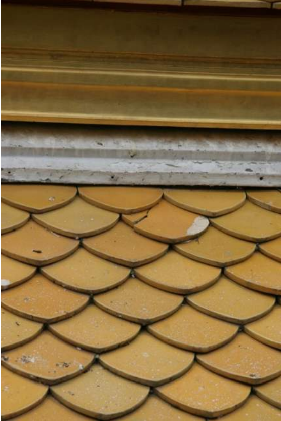
Thai Pavilion roof detail condition.
