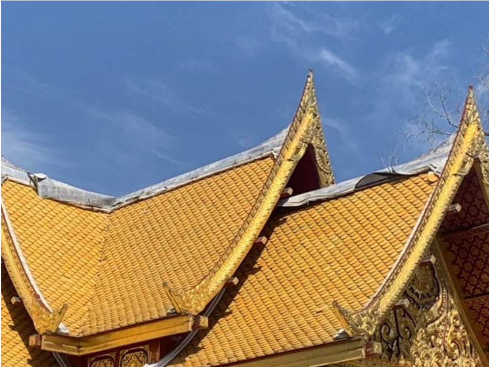
Condition of Thai Pavilion ridge cap.
