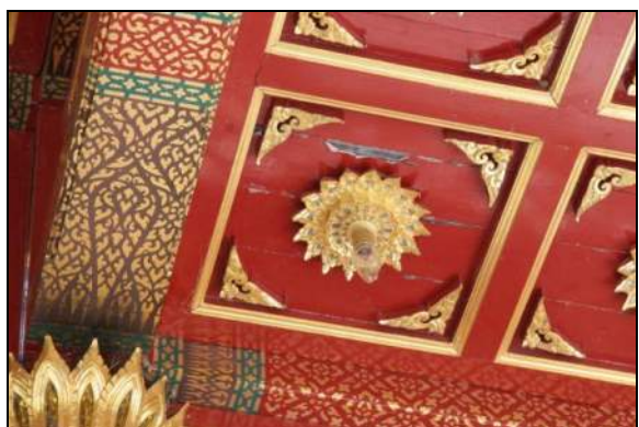
Fig. 11 – peeling paint inside – sala ceiling
