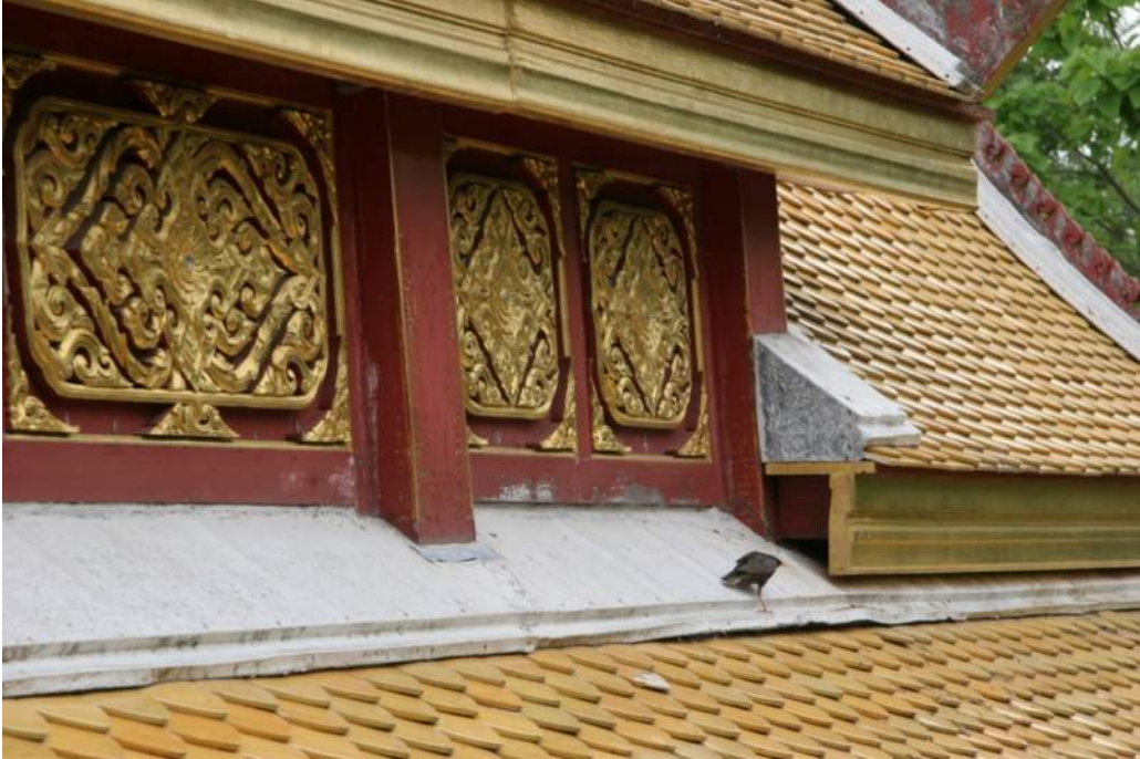
Thai Pavilion roof detail condition.
