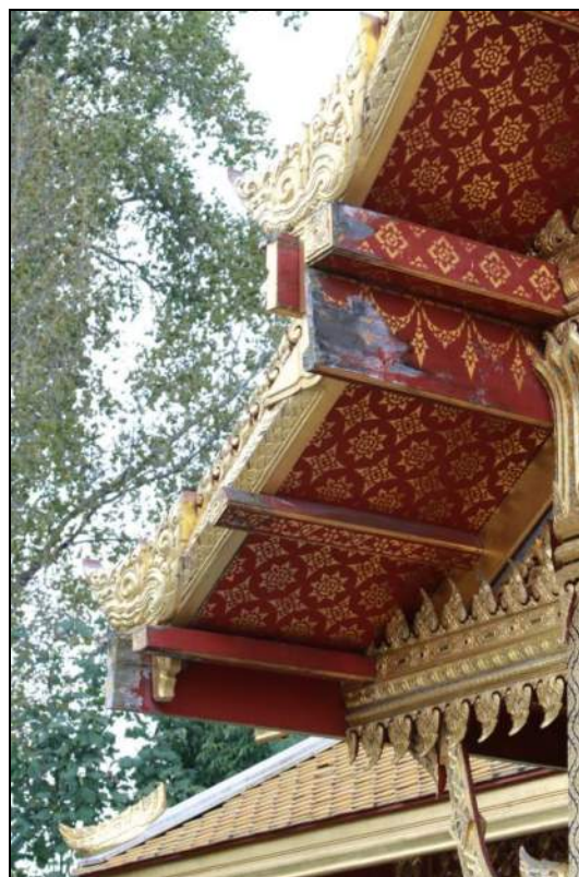
Fig. 21 – wood splitting on west gable end
