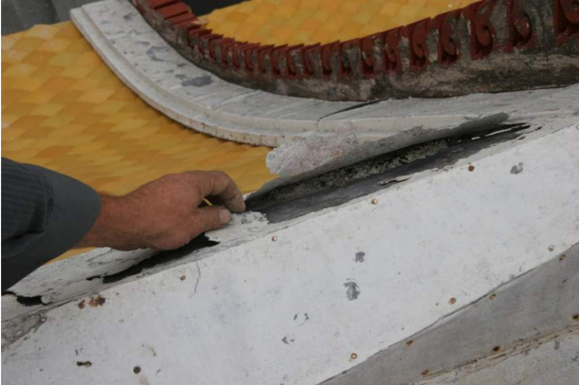
Thai Pavilion ridge cap condition 2016.
