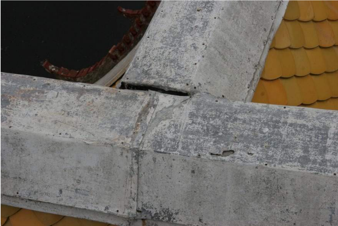
Thai Pavilion ridge cap condition 2016.
