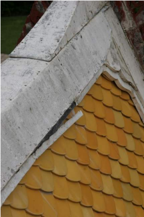
Thai Pavilion roof detail condition.
