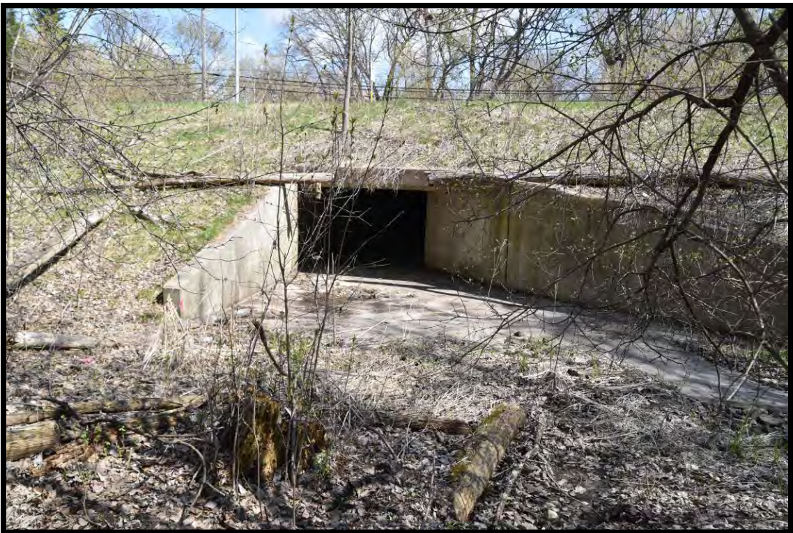
Figure 14: View to northeast of existing culvert on the southern side of University Avenue.
