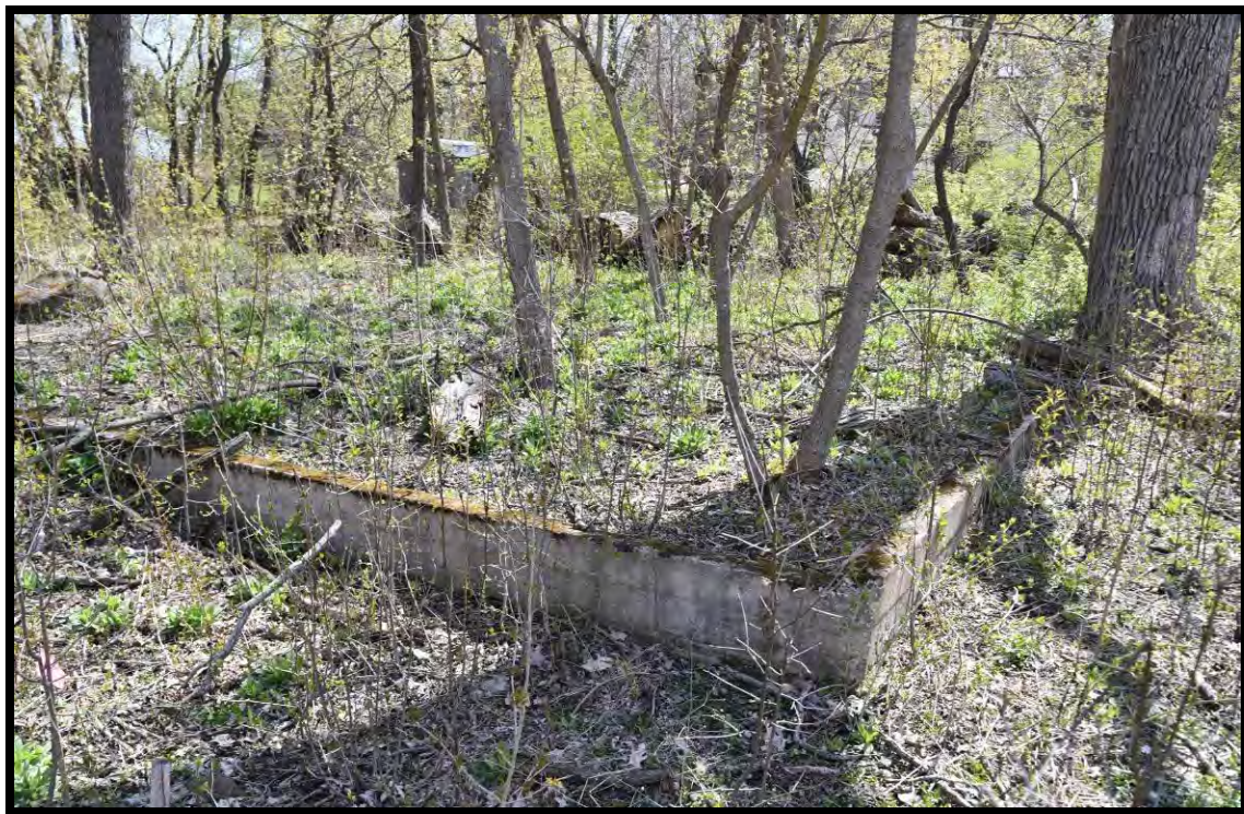
Figure 24: View to south of foundation identified during field investigation and recorded by SHSW as DA-1604.
