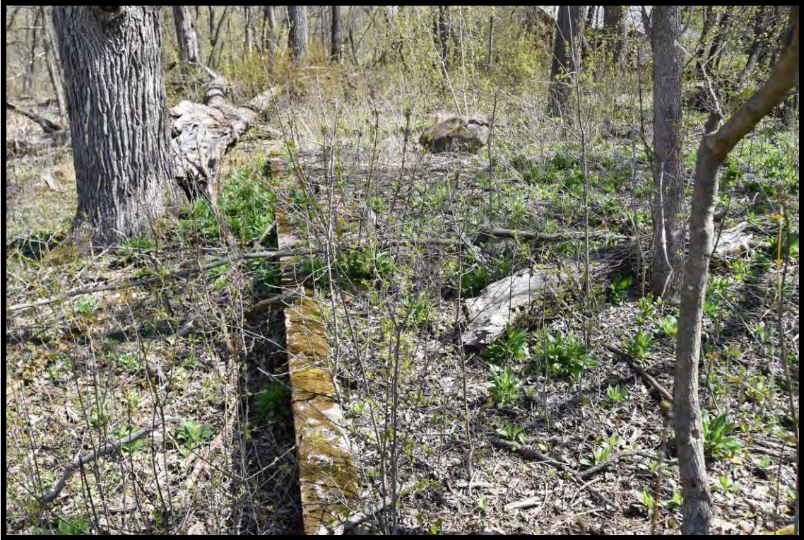
Figure 13: View to north of northwest corner of building foundation reported as DA-1604.
