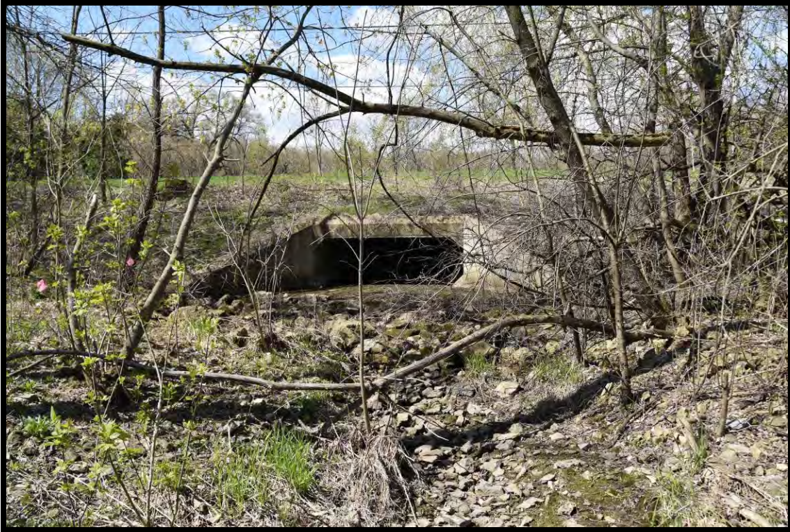
Figure 9: View to southwest area of existing culvert at the central terminus of Project at Old Middleton Road.
