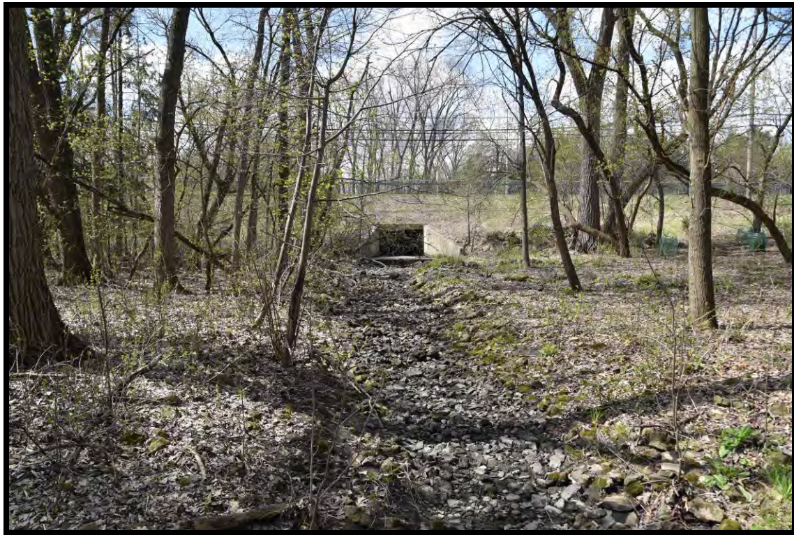
Figure 15: View to southwest of existing culvert on the northern side of University Avenue
