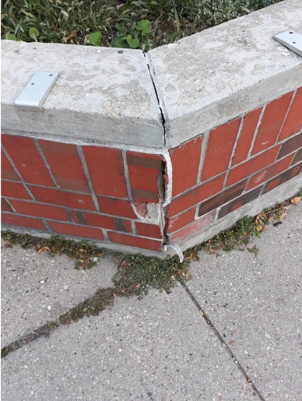
CSN 4: Damaged Planters
