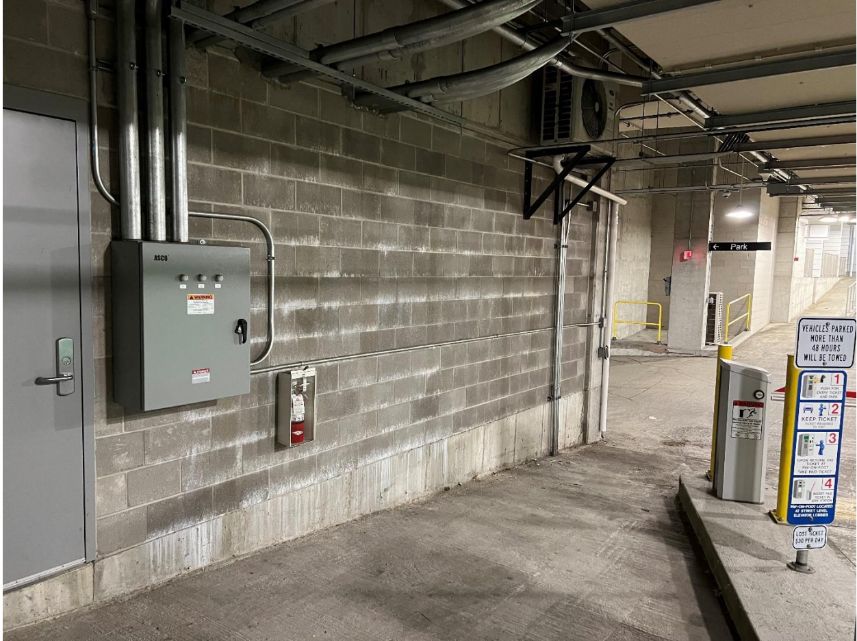
WSG 2: Efflorescence of CMU Wall at Level 1
