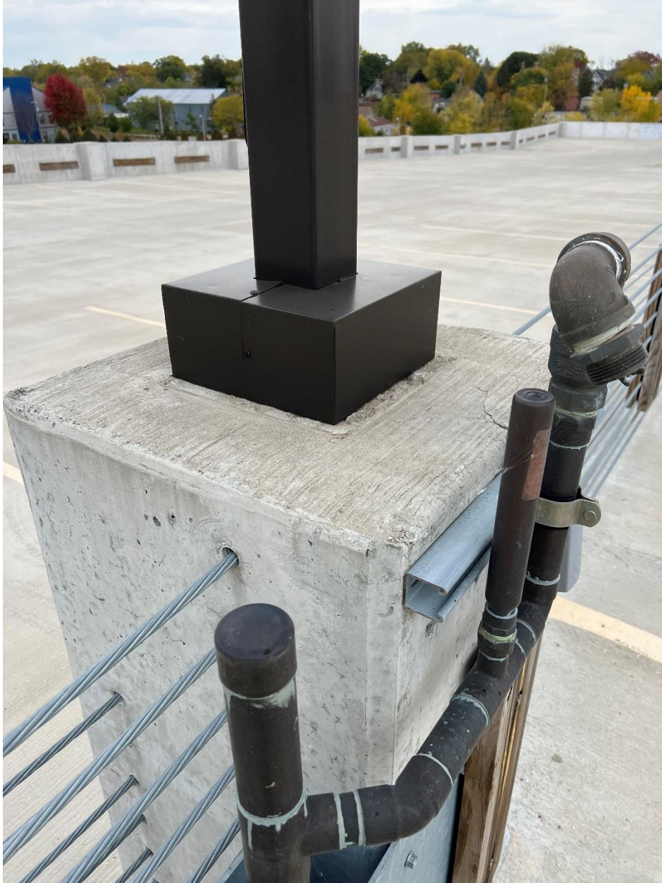
SLS 1: Missing Sealant at Roof Light Pole Bases
