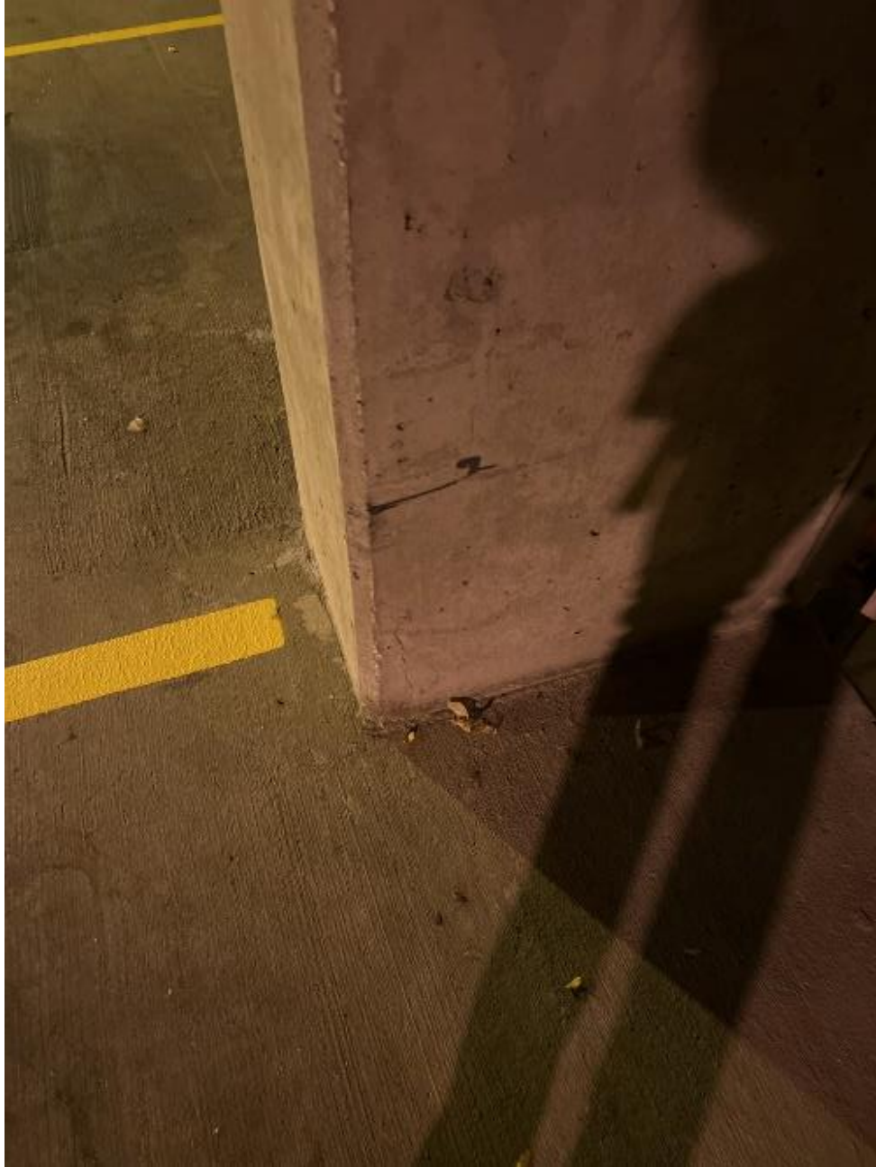
OC 2: Spalled Column
