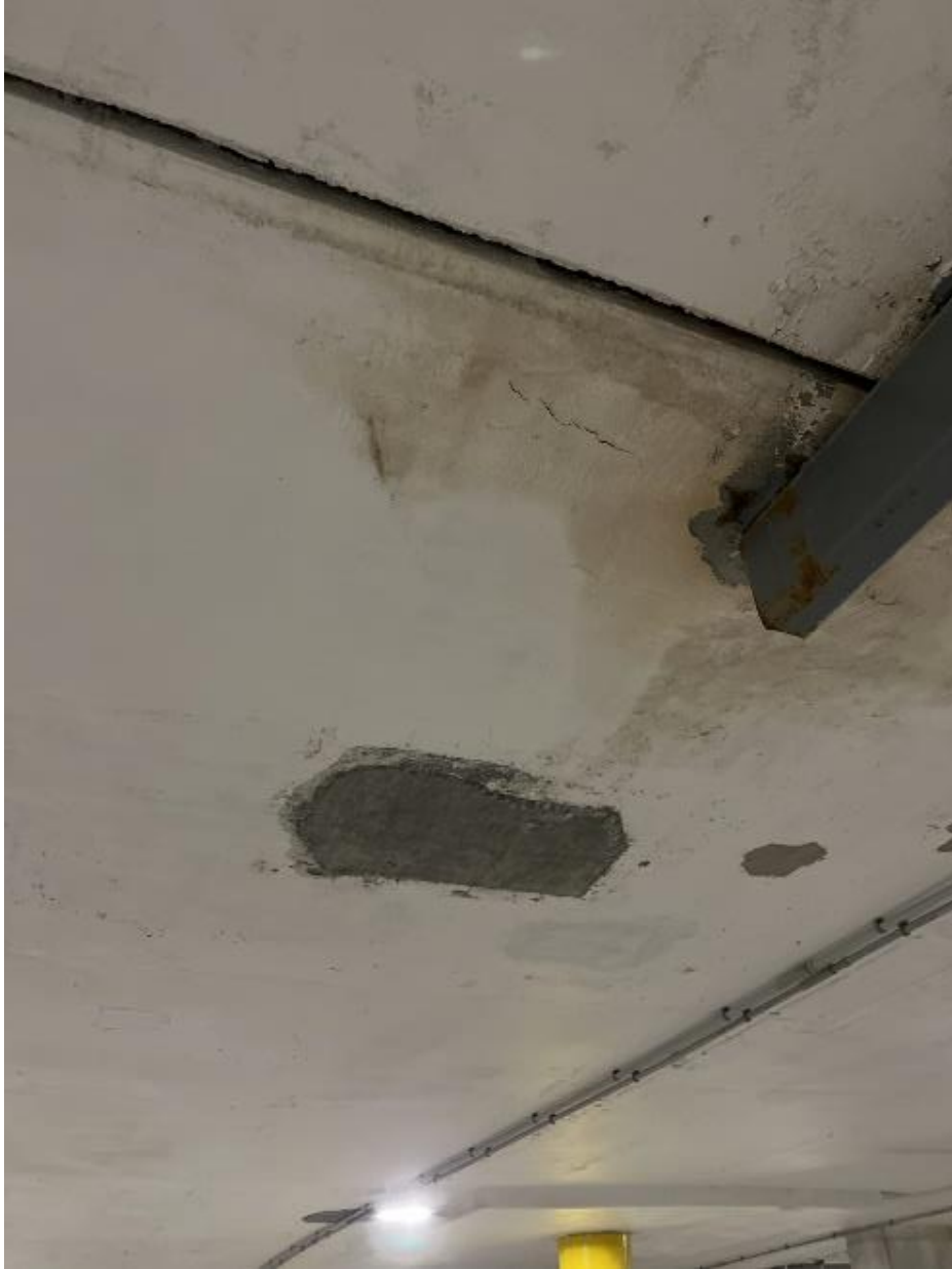
SSCo 1: Spalled Slab
