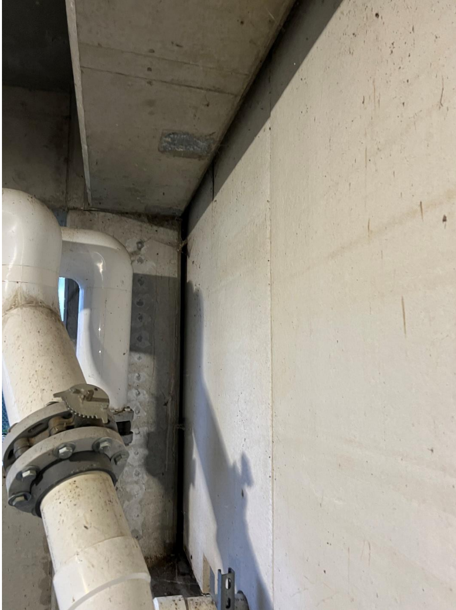
SLS 2: Misaligned Precast to Beam and Knee Wall Embeds (Level 1)
