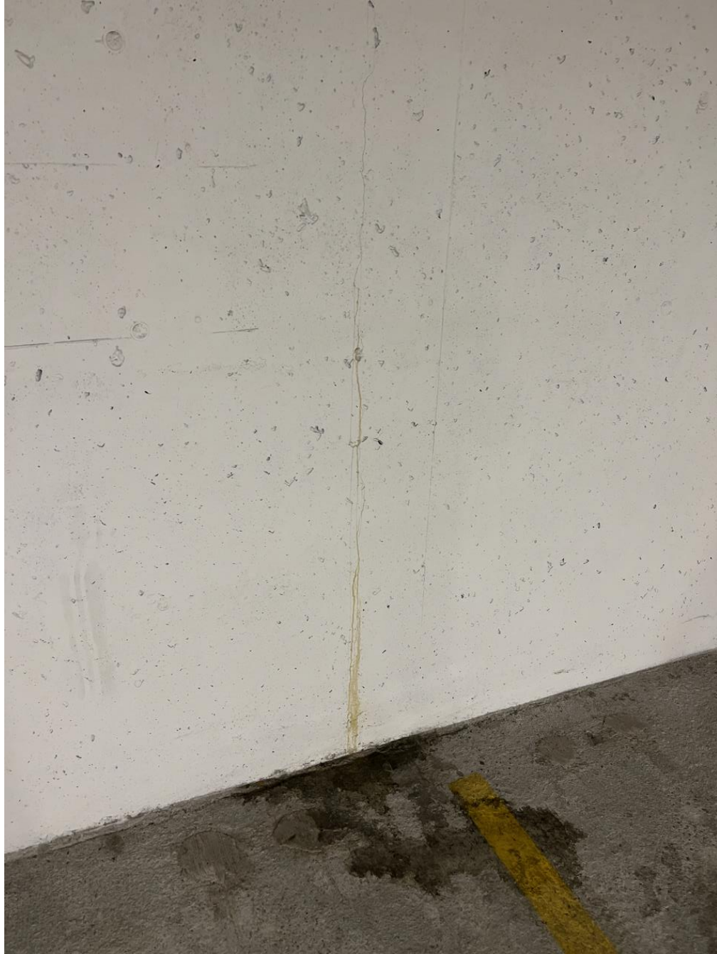
WSG 1: Active Leak in Foundation Wall
