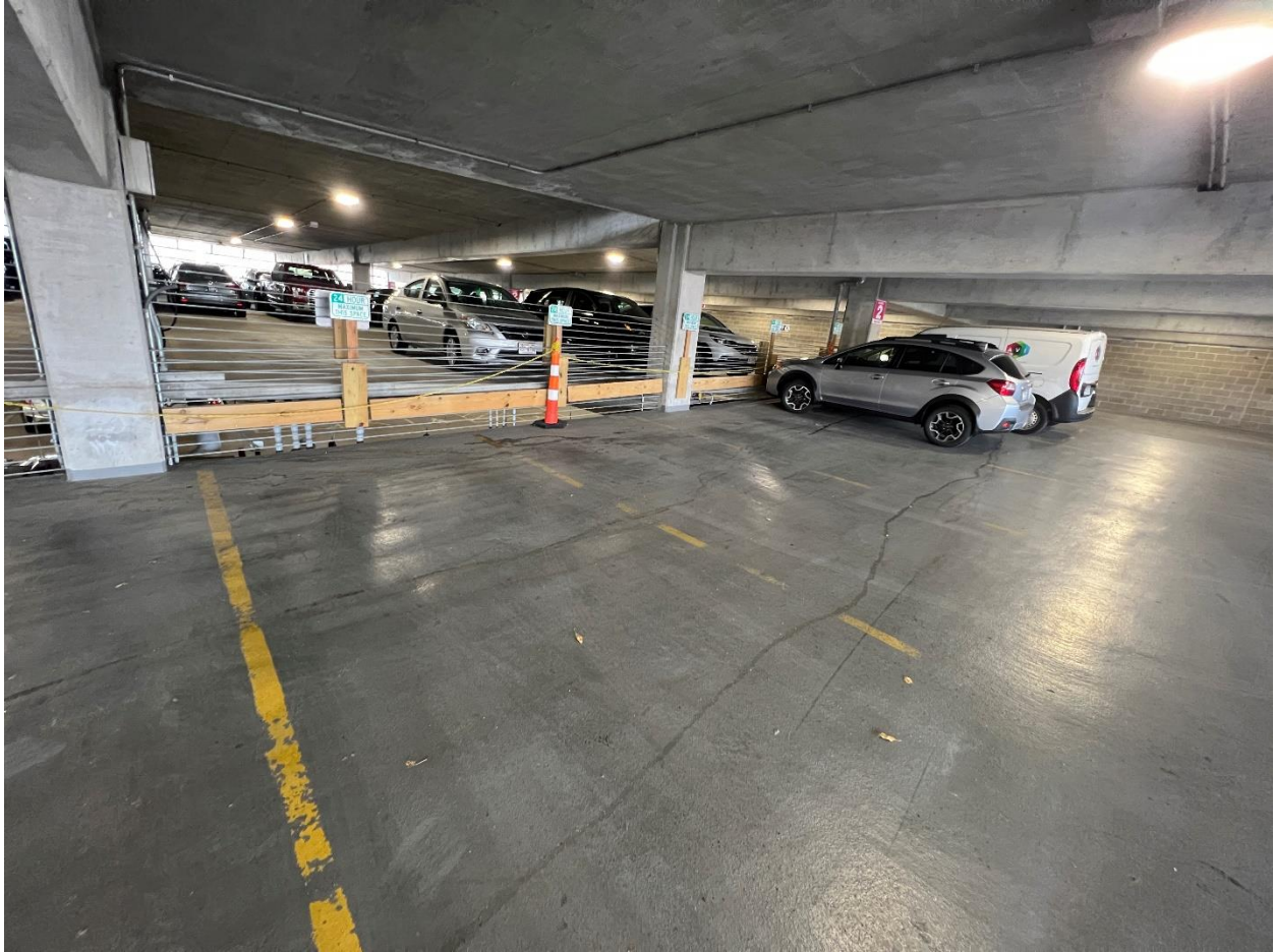
SLS 5: Worn Striping at Interior Parking Stalls on Level 2 Ramp
