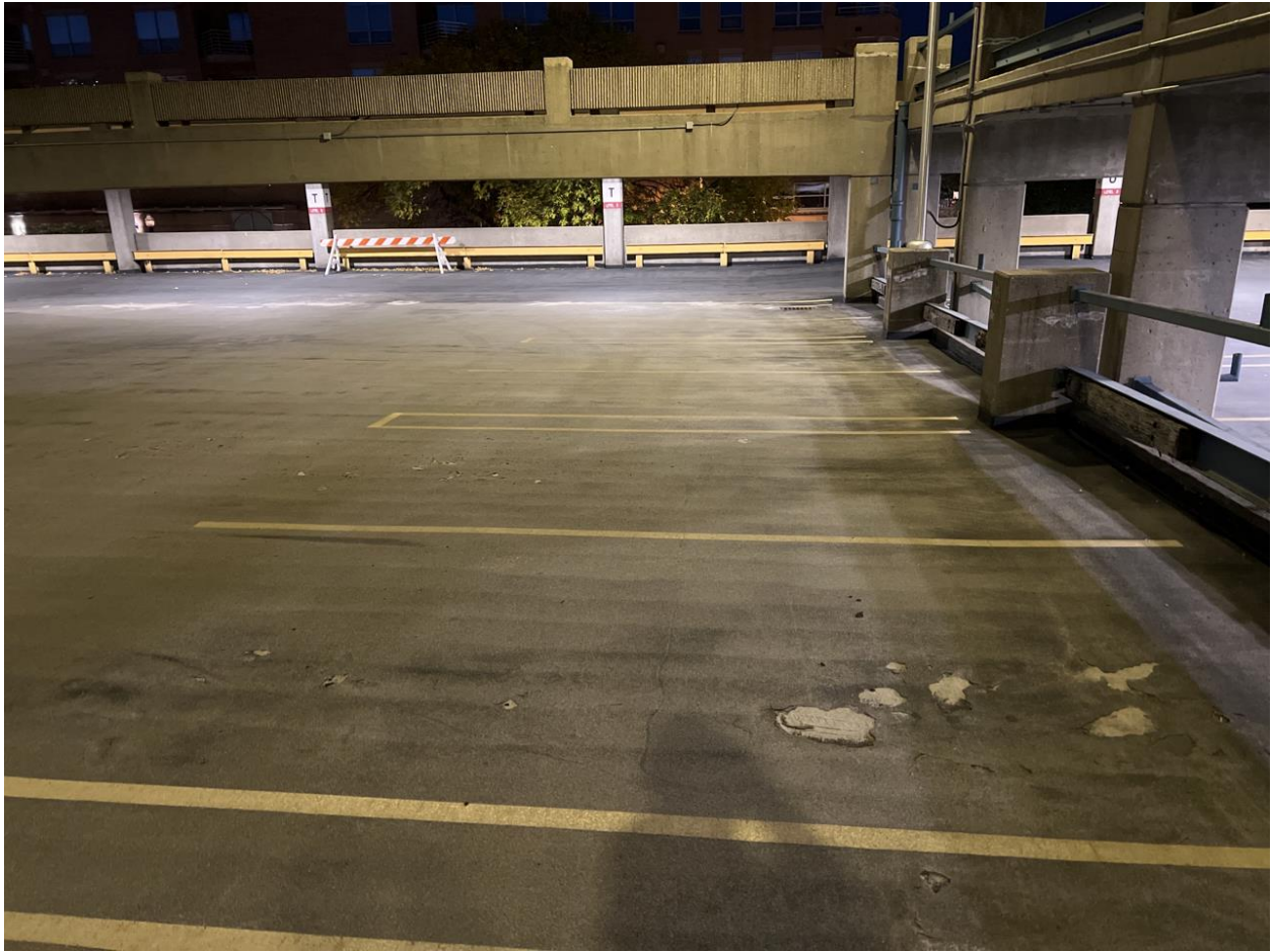
CSN 7: Poor/Failed Membrane Condition at Roof
