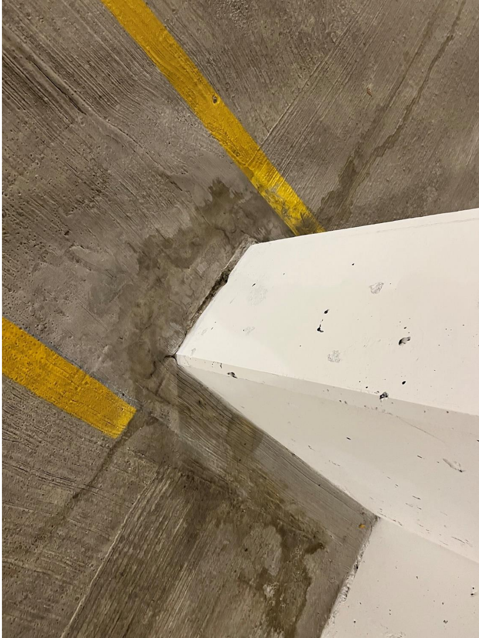
WSG 3: Unsealed Interior Ramp Columns
