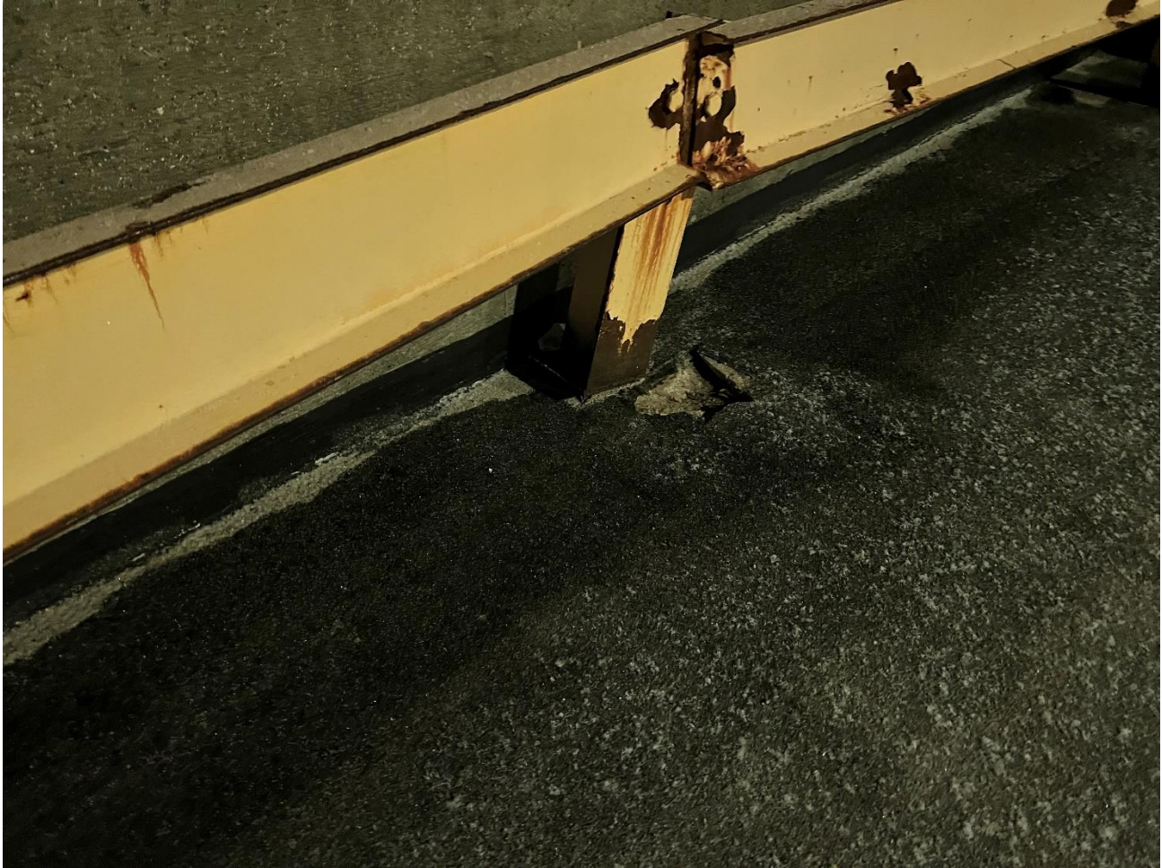
CSN 6: Damaged Roof Barrier Steel
