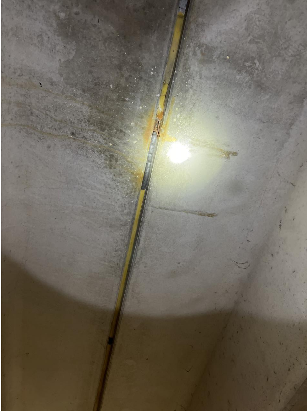
SSF 2: Corroded Precast Double Tee Shear Connector (Overhead)
