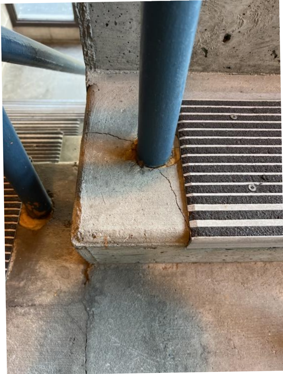
OC 4: Spalled Slab
