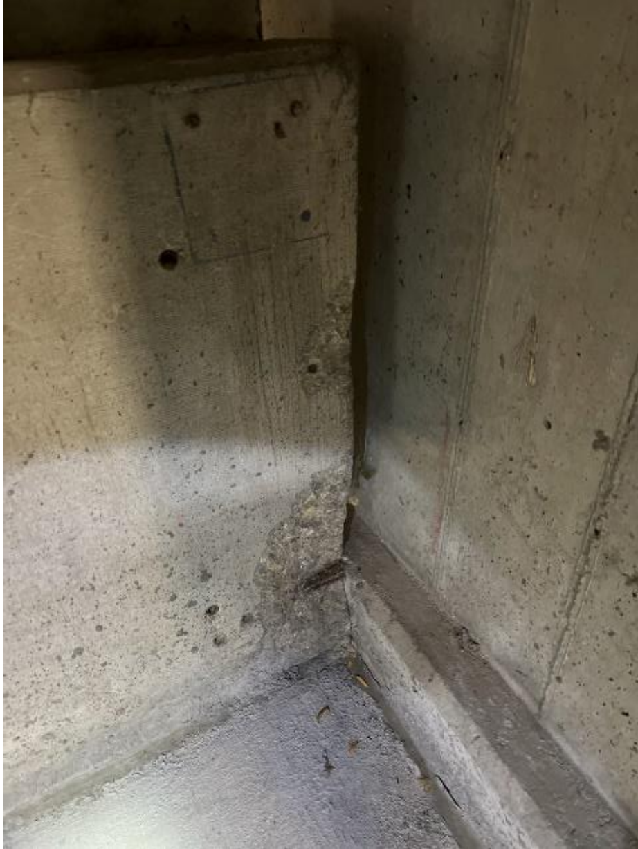
SSCo 2: Spalled Wall
