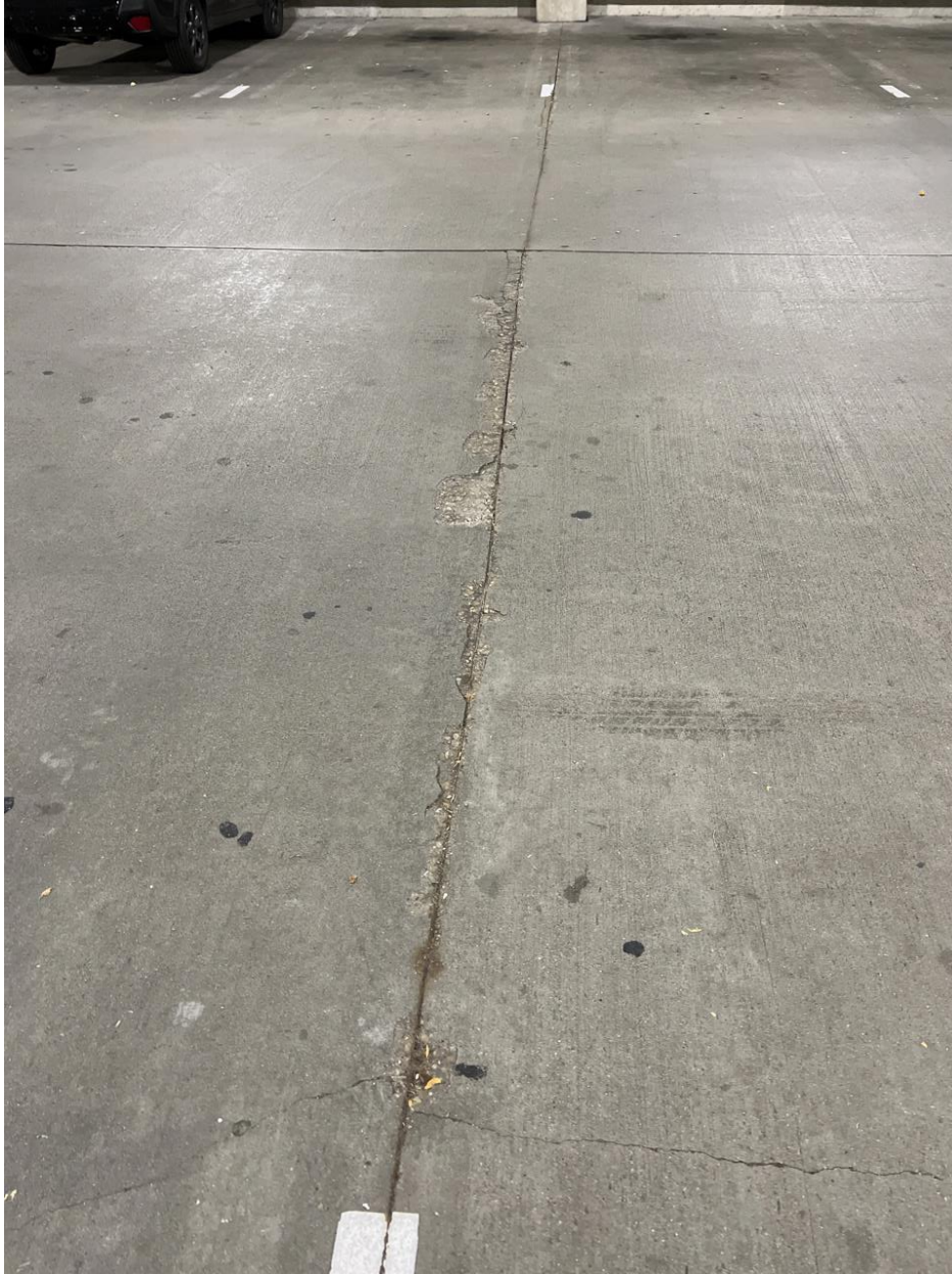
CSN 3: Spalling at Slab on Grade Joints
