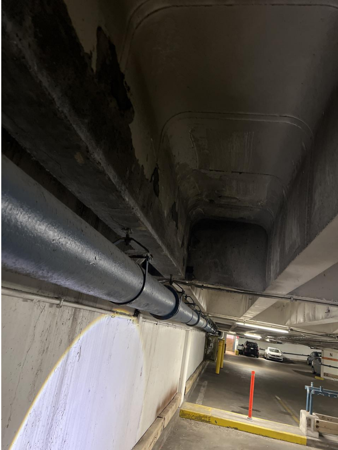
SSL 2: Joist Spall at Existing Repair with Embedded Pipe Hangers
