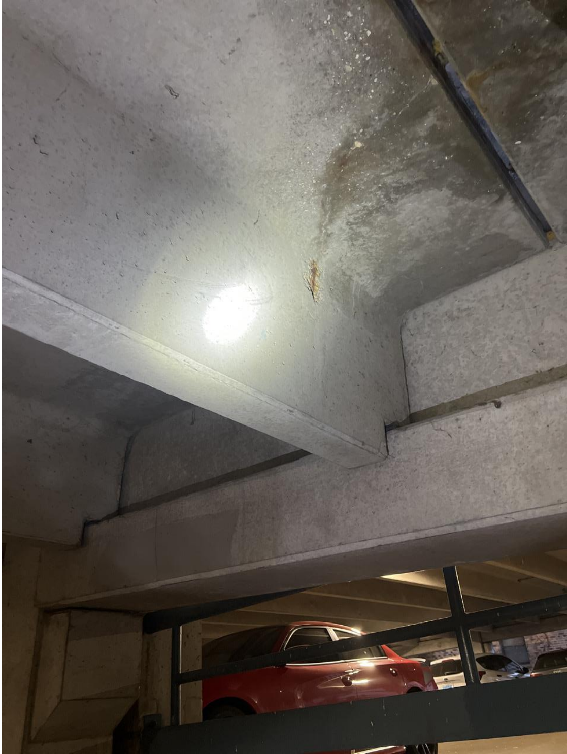
SSF 1: Exposed Corroded Bar on Double Tee Stem
