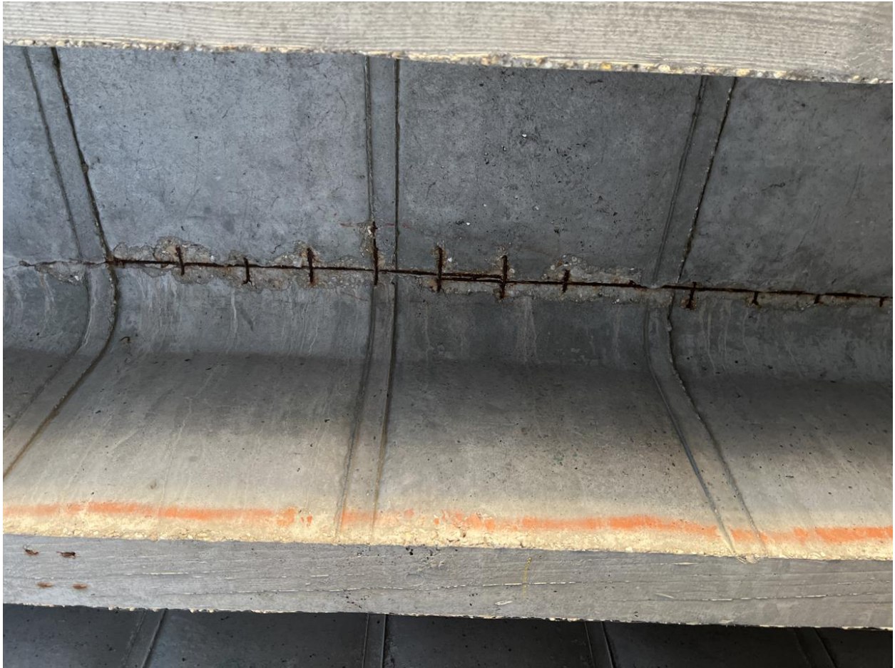
SSL 1: Corroded Exposed Bars in Slab Crack (Overhead)
