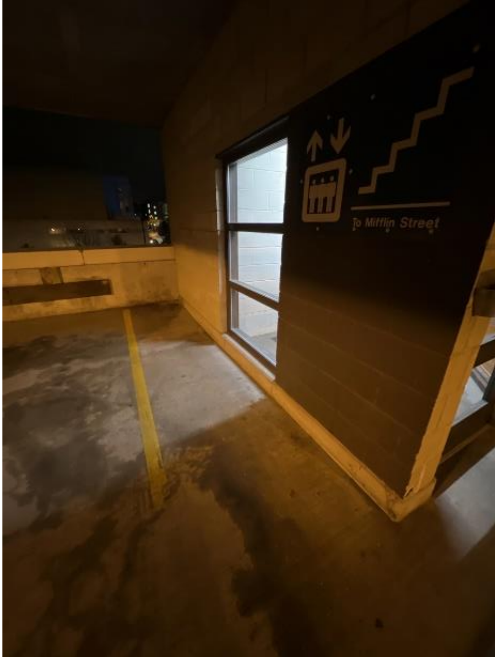
OC 1: Failed Sealant Joint
