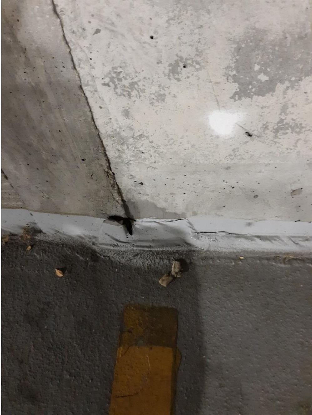
SSCo 5: Failed Sealant Joint
