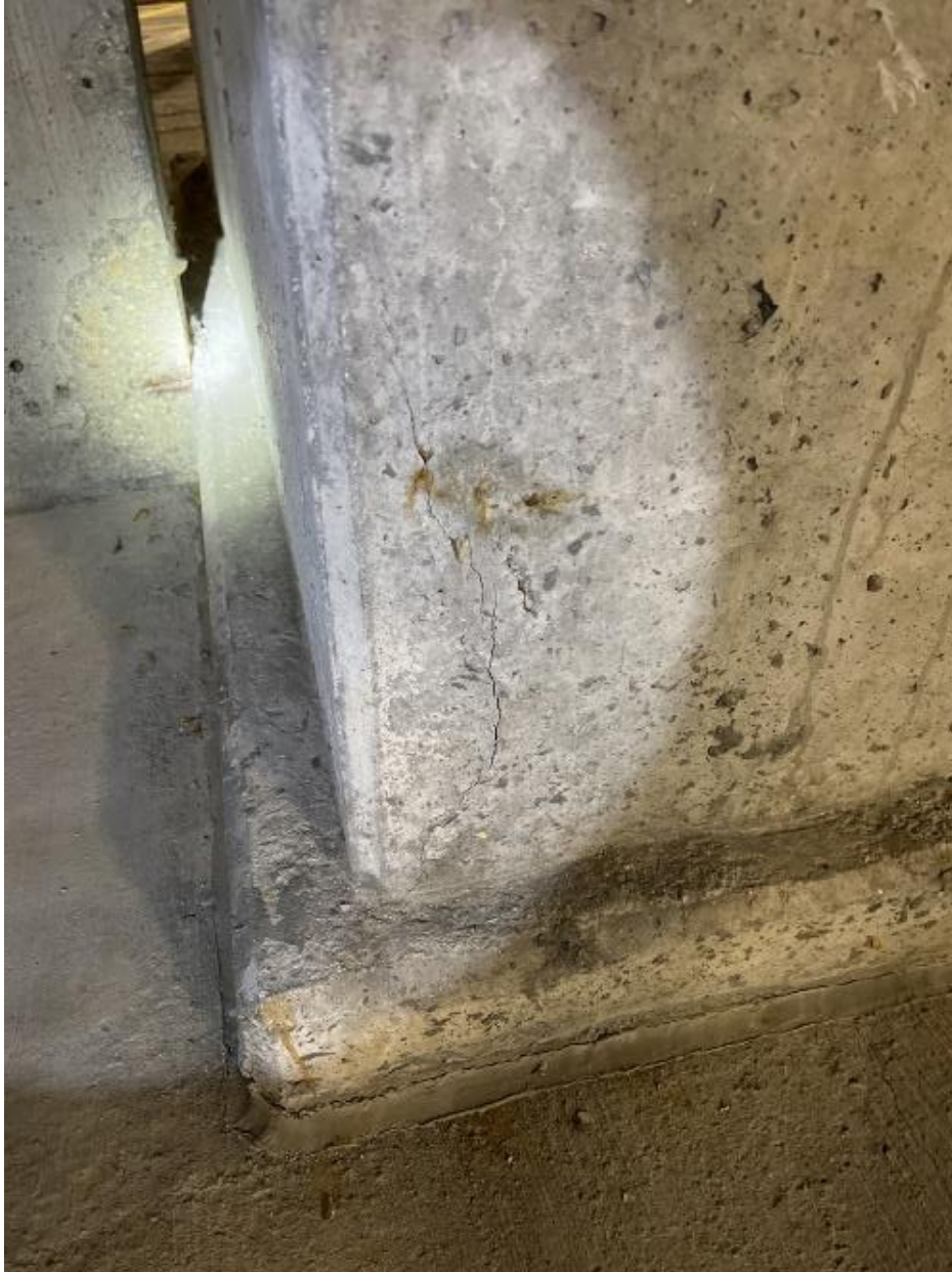
SSCo 3: Spalled Column
