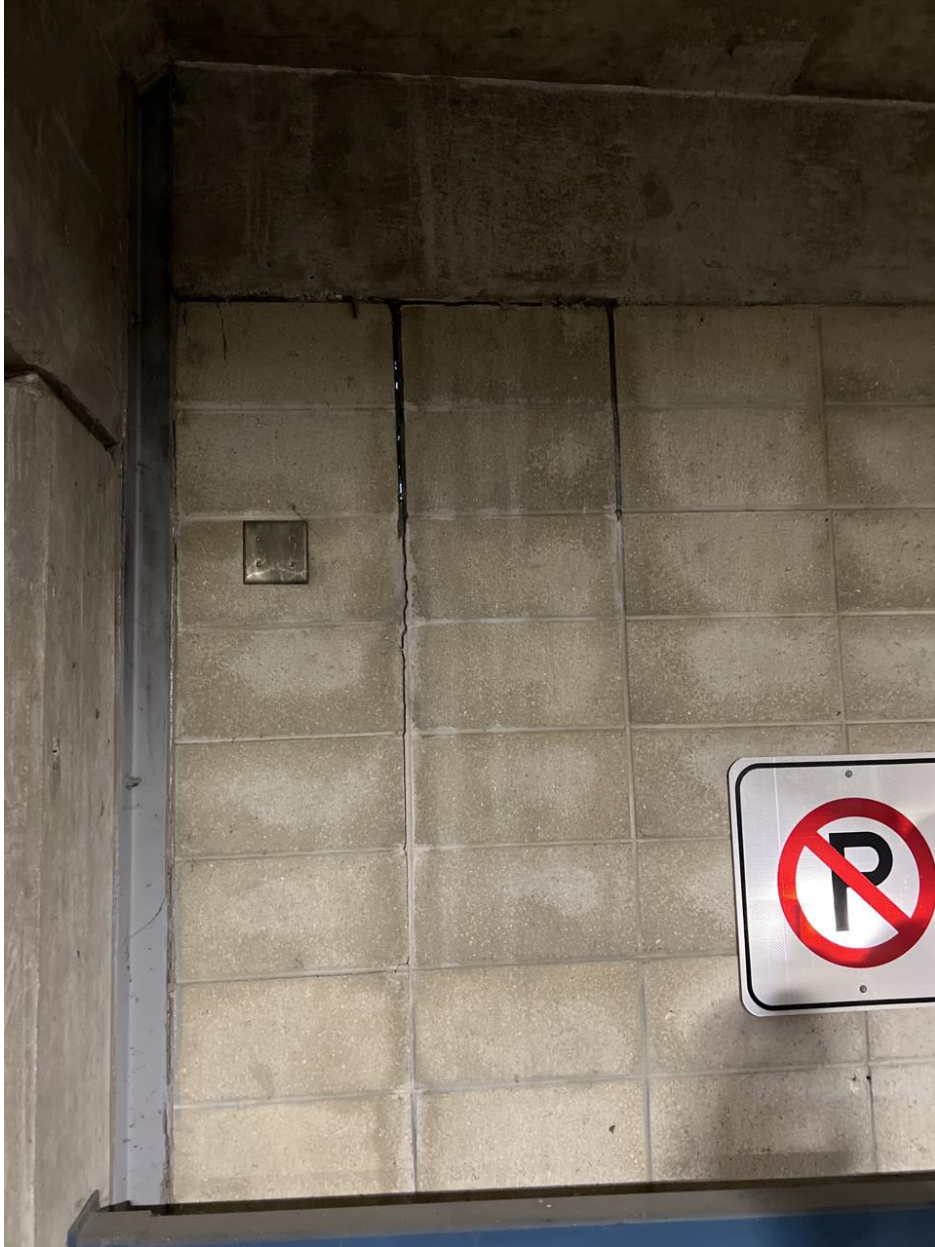
CSN 1: Failed CMU Vertical and Head Joints
