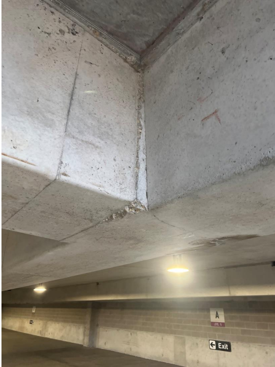
SSCo 4: Spalled Beam
